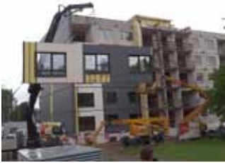
Installation of a prefabricated module for building renovation in a pilot project in Tallinn. Source: Technical University Tallinn
